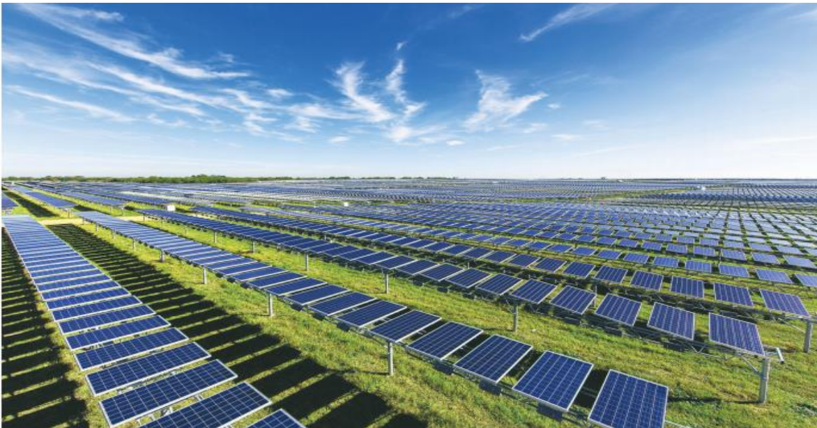
Figure 9-- Alamo 4 Solar Installation, CPS Energy utility-scale project
