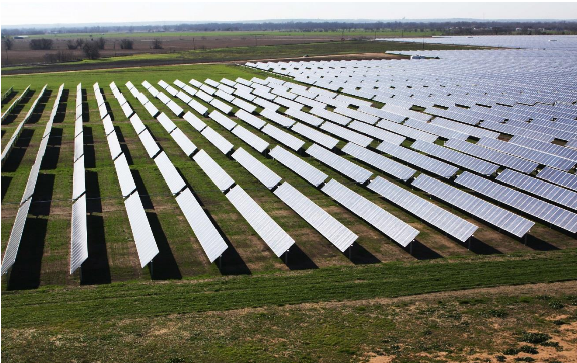
Figure 1-- Austin Energy Solar Installation
