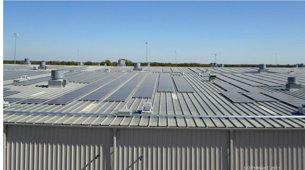
FedEx Hub, Hutchins, Texas. Largest rooftop PV system in N. Texas (~1.4 MW)
